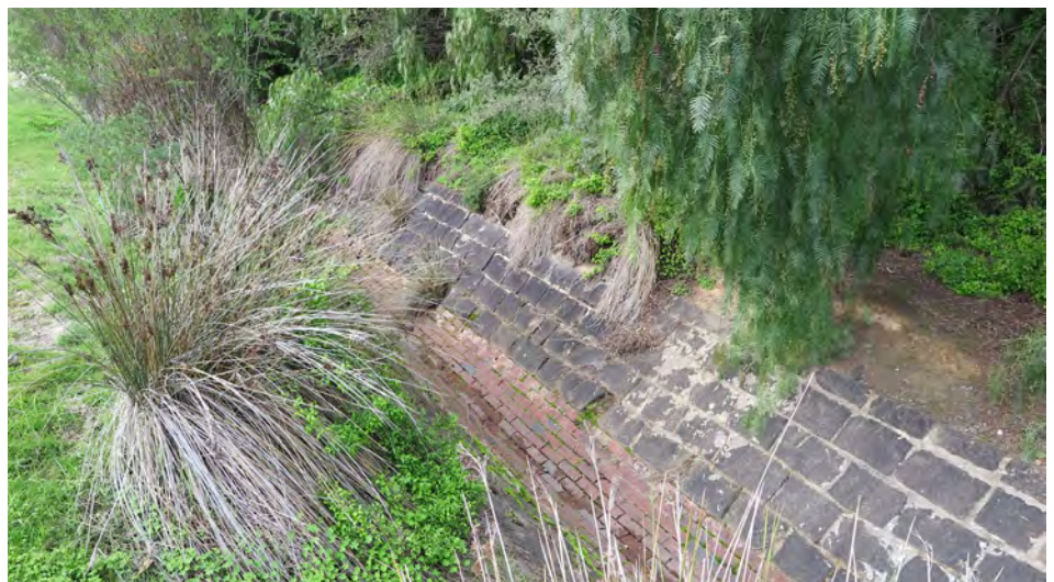
This section of V-drain is flanked by a stand of peppercorn trees at the Garden Gully Reserve. Tree roots are causing damage to sections of the drain.
