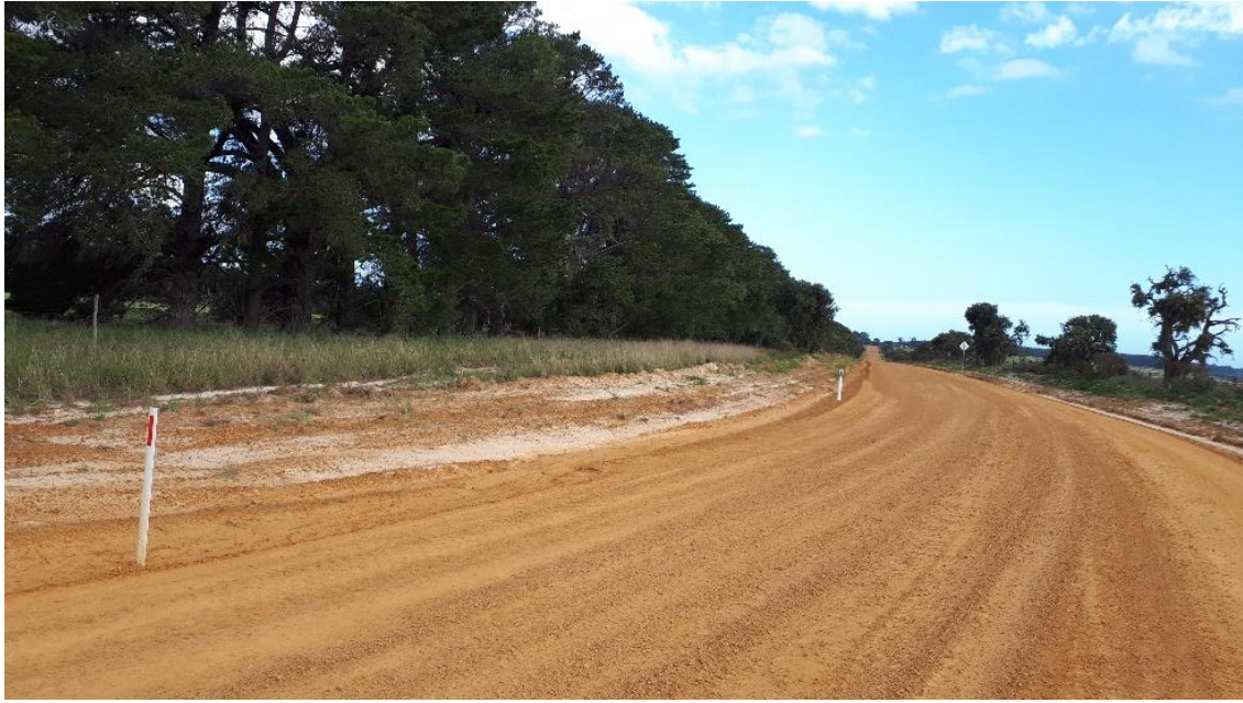
Figure 11. Evidence of completely destroyed sections
